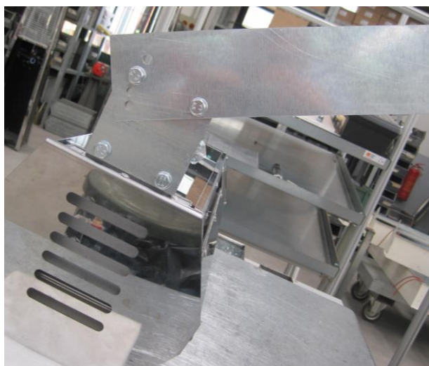
picture 1 – Installation at wall D-RAD
